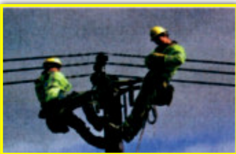
Fig (2-18): Electricity is safe if it is handled cautiously
