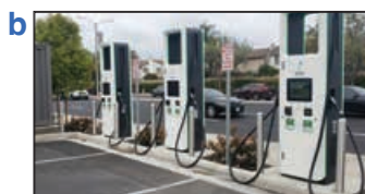
b charging station
