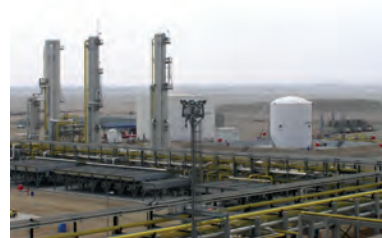
Water purification station
