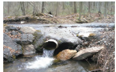
Discharging sewage in canals
