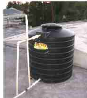
Water tank Figure (16)
