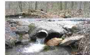
Discharging sewage in canals
