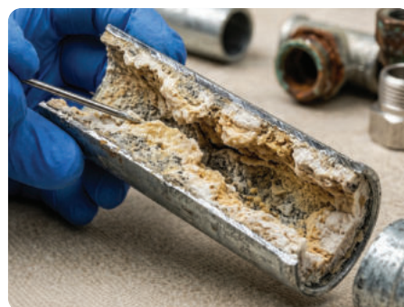
Figure (23) Hard deposits inside water pipes
